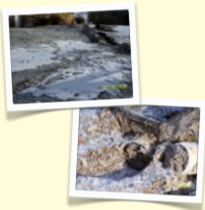
Top photo: Real Property Transfer Inspection (Barrington) Bottom photo: Distribution box was plugged with mouse nest and silt
