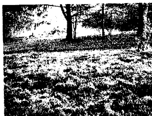
Failed system detected in an evaluation of a system. System at times was surface discharging to a ditch.
